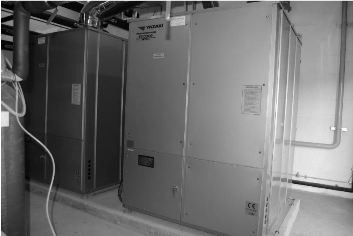
Figure 5: The cooling station
