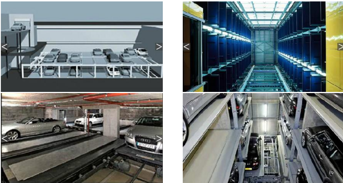
Fig. 5. Application of automated parking systems (Techno Team System)
