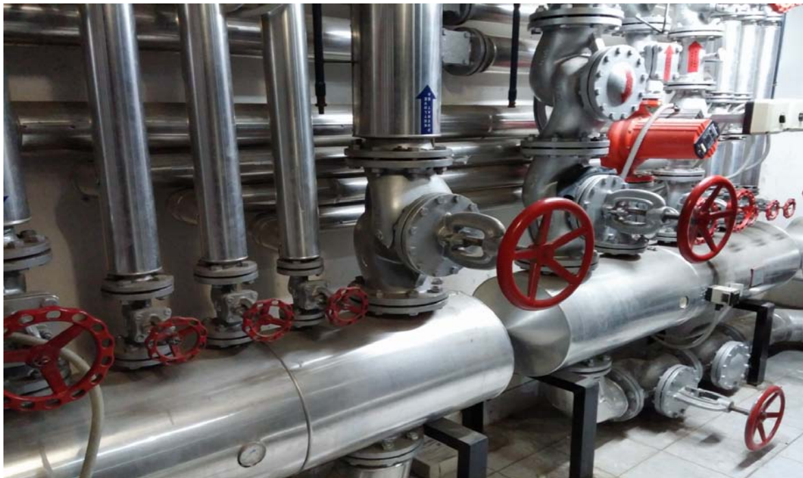
Picture 4. Existing machinery room in hotel „Berulia“
