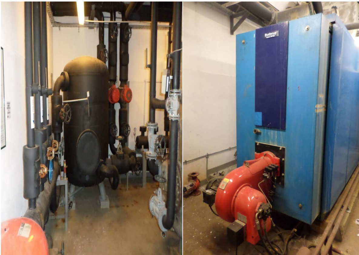
Picture 3. Existing machinery room in hotel “Maestral”
