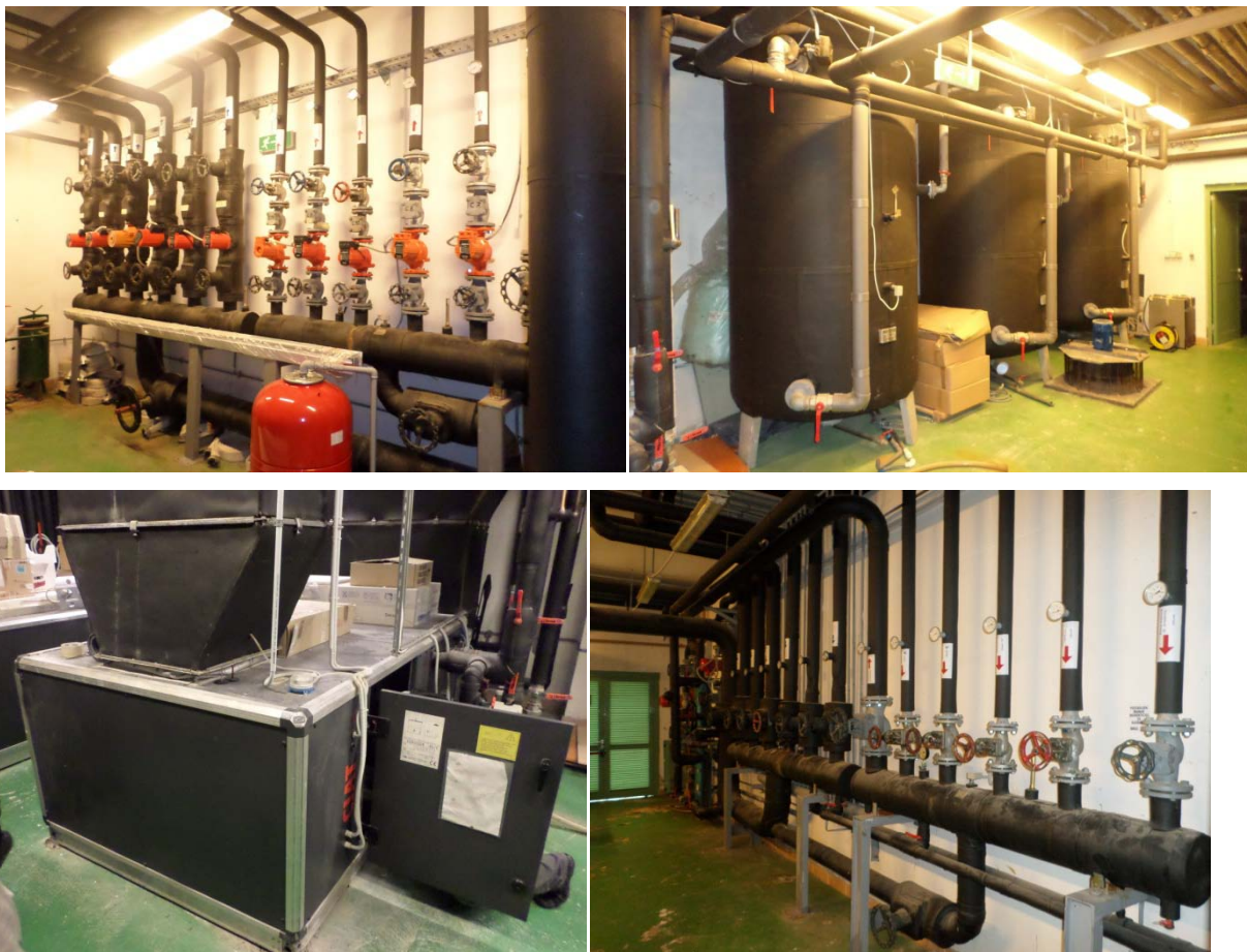
Picture 5. Existing machinery room in hotel "Marina"
